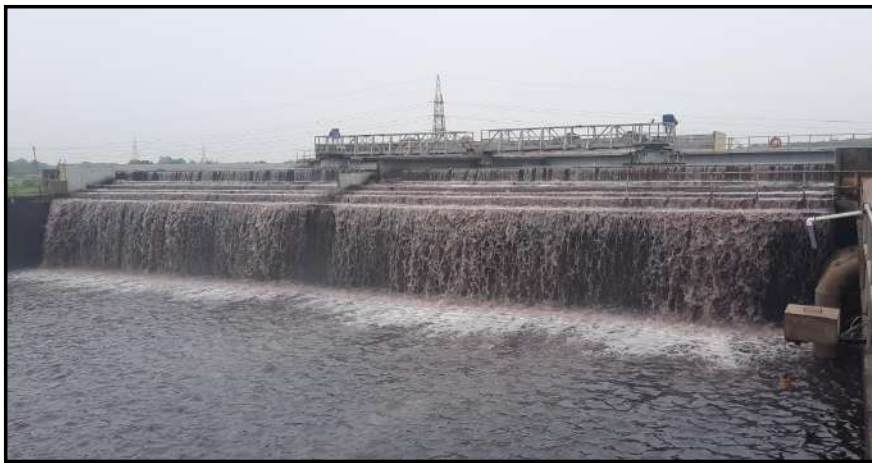
Fig. 3.3 New Cascade Cooling System at CETP
