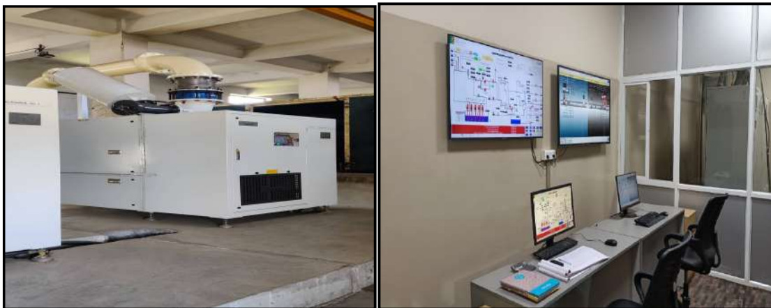
Fig 3.7 a) Centrifugal Turbo Blower and b) SCADA- PLC control Room
