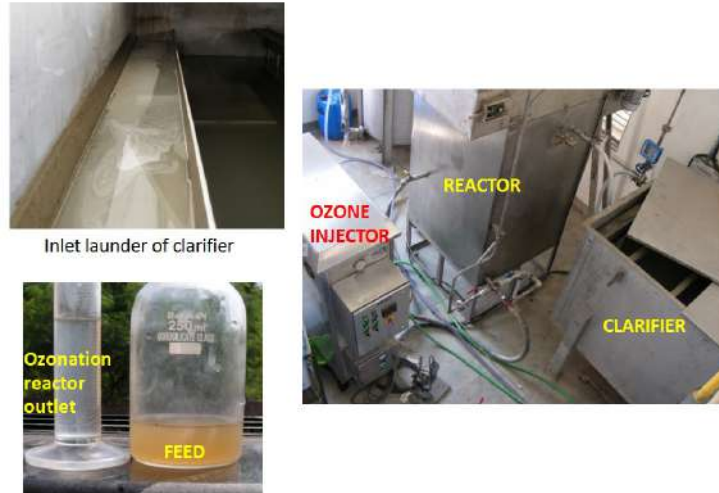
Figure 7: Photograph of AEWTP in operation.
