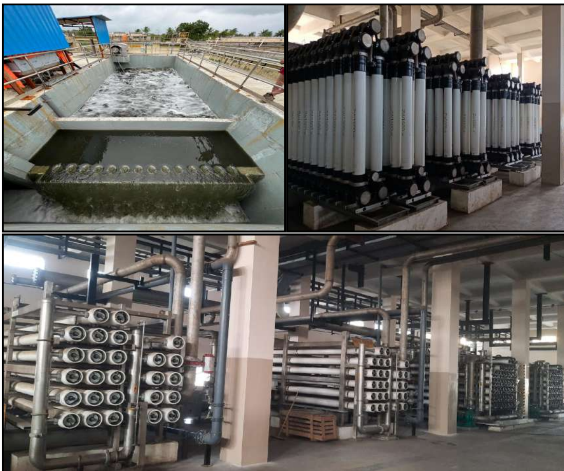
Figure 3.8 a) New Fibre Disc Filter System b) Ultrafiltration Plant C) Reverse Osmosis Plant
